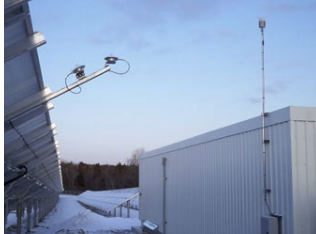
This weather station installation shows the two radiation sensors, one at plane of array and one at GHI, as well as the Orion weather sensor module on the mast. MicroServer and Acromag amplifier are in the weatherproof enclosure mounted below the mast. Photo courtesy of Industrial Electrical Contactors Ltd.
