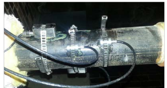
Clamp-on PT100 transducers fixed to pipe as used by PA Energy
