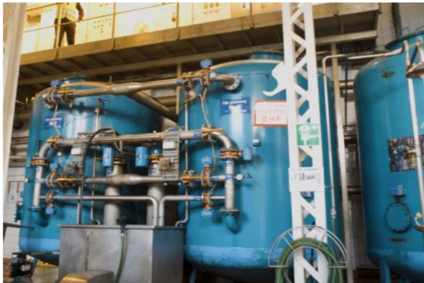
This hydrophore system maintains stable water pressure at the Carlsberg brewery.
