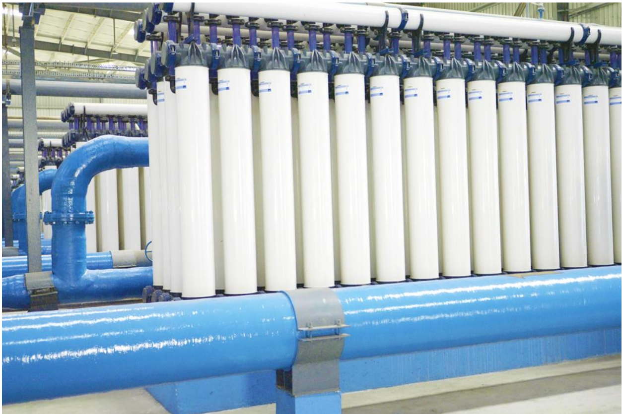
Reverse osmosis technology is increasingly used in wastewater treatment.
